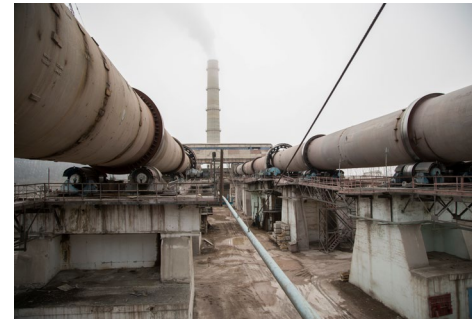
Kilns in Cement and Cement Product Manufacturing
