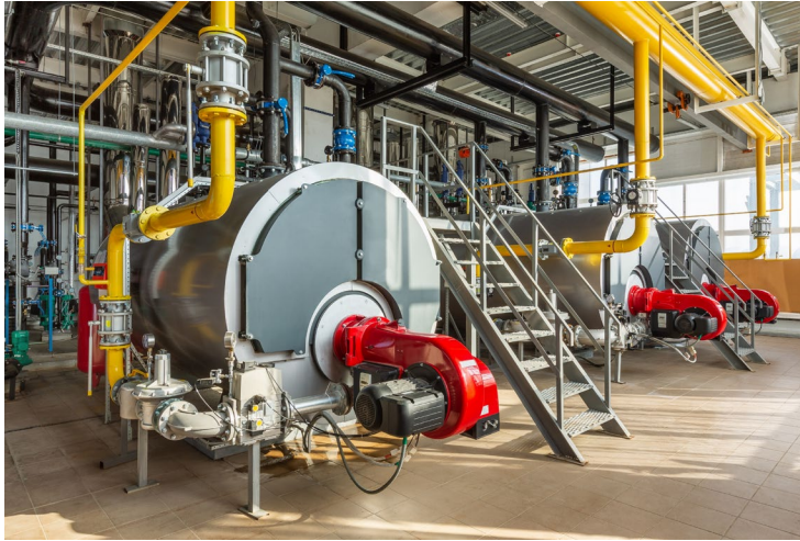
Boilers in Iron and Steel Mills and Ferroalloy Manufacturing, Metal Ore Mining, Basic Chemical Manufacturing, Petroleum and Coal Products Manufacturing, and Pulp, Paper, and Paperboard Mills
