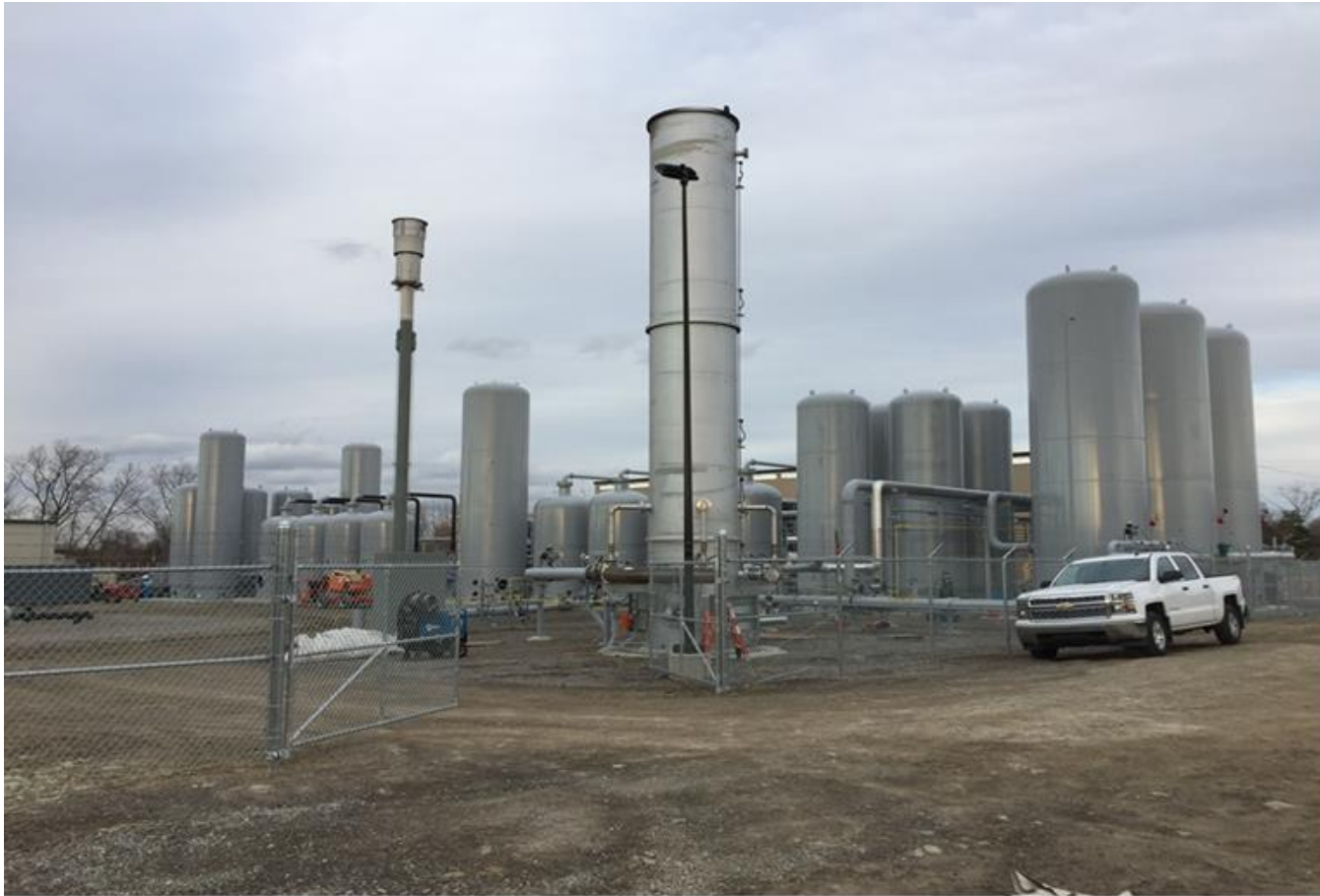
Landfill Gas to RNG Facility, Michigan
